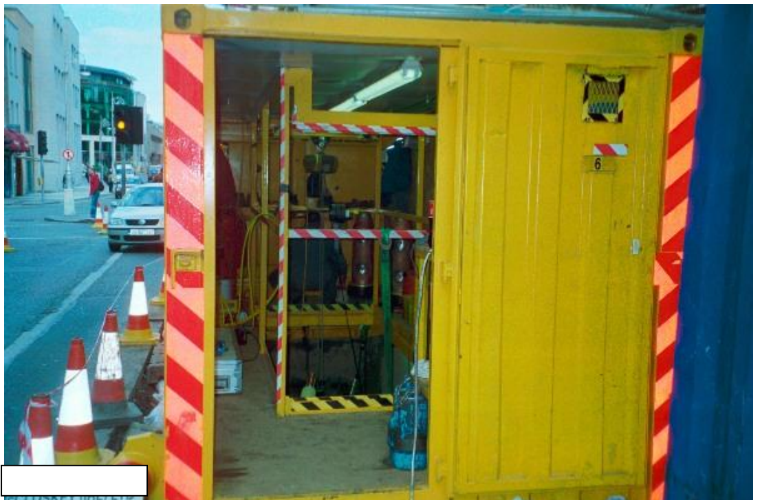
Plate 9 : HV cable jointing container
